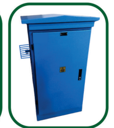
Street Light Control Panel
